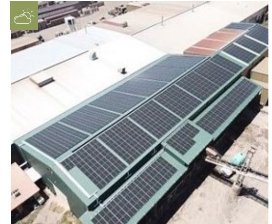
CSR PGH Cecil Park, NSW manufacturing facility
