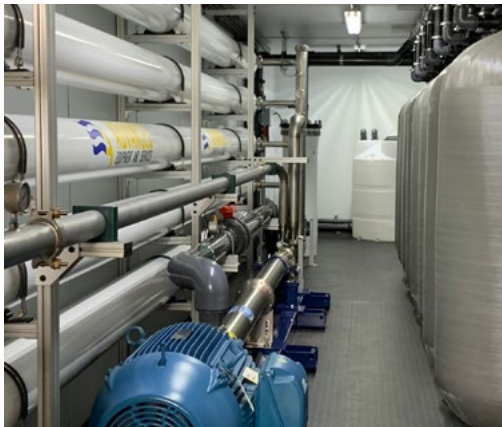
CSR's Brendale water treatment plant in QLD
