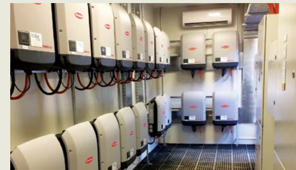
SOLAR INVERTER ROOM, GOLDEN GROVE
