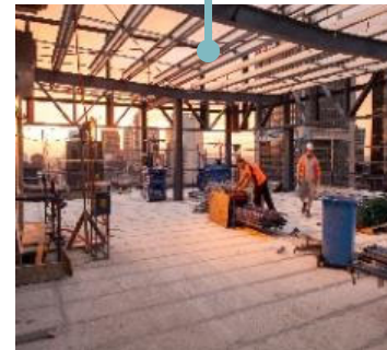
Commercial flooring systems complement design flexibility of steel structures
